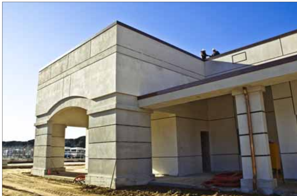
Navy and Defense Commissary Agency engineers inspect the construction on the new Camp Darby commissary. DeCA hopes to take beneficial occupancy of the facility in March and open in May.
